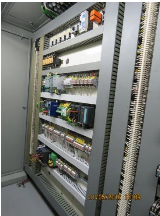
Figura 4. Tablero remoto instalado dentro del TIC (RRTIC).
